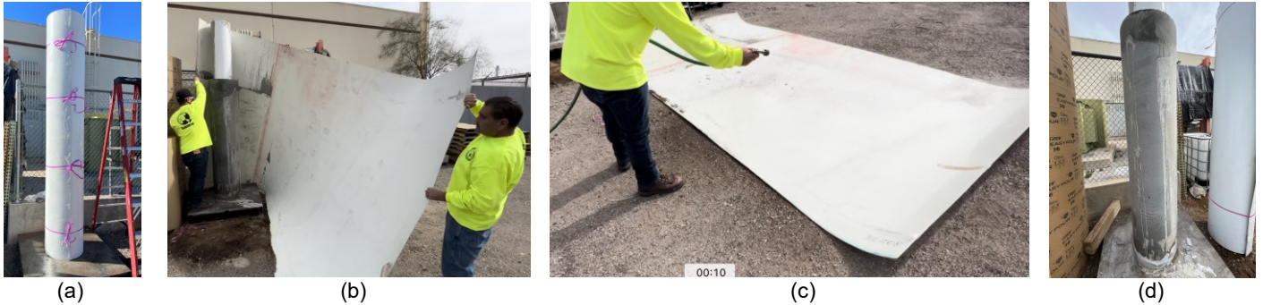
Fig. 3. Field application: (a) FLF placed and filled with concrete, (b) removing the laminate after concrete hardens, (c) cleaning and saving the laminate for future use, and (d) smooth concrete finish with no spiral marks
