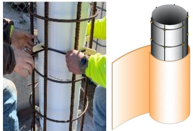
Fig. 2. Spacers being installed and the FLF laminate being wrapped around a deteriorated column
