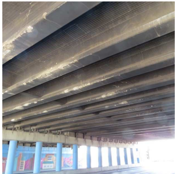
Fig. 3. Damage to 19 th Ave. bridge girders from numerous collisions.
