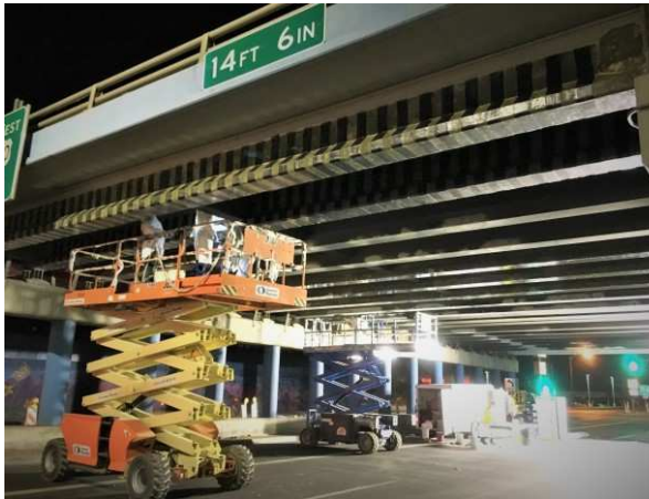
Fig. 8. Installation of CFRP strips on the 11 girders at the 19 th Ave. bridge.
