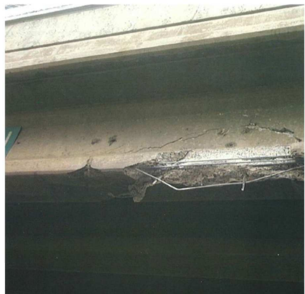
Fig. 2. Damage to Jefferson Street underpass from one of the earlier collisions.
