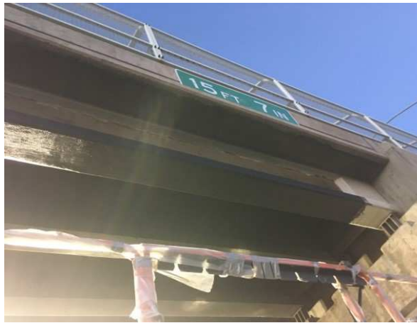
Fig. 6. Location of the severely damaged girder and CFRP repairs at Jefferson St. bridge.
