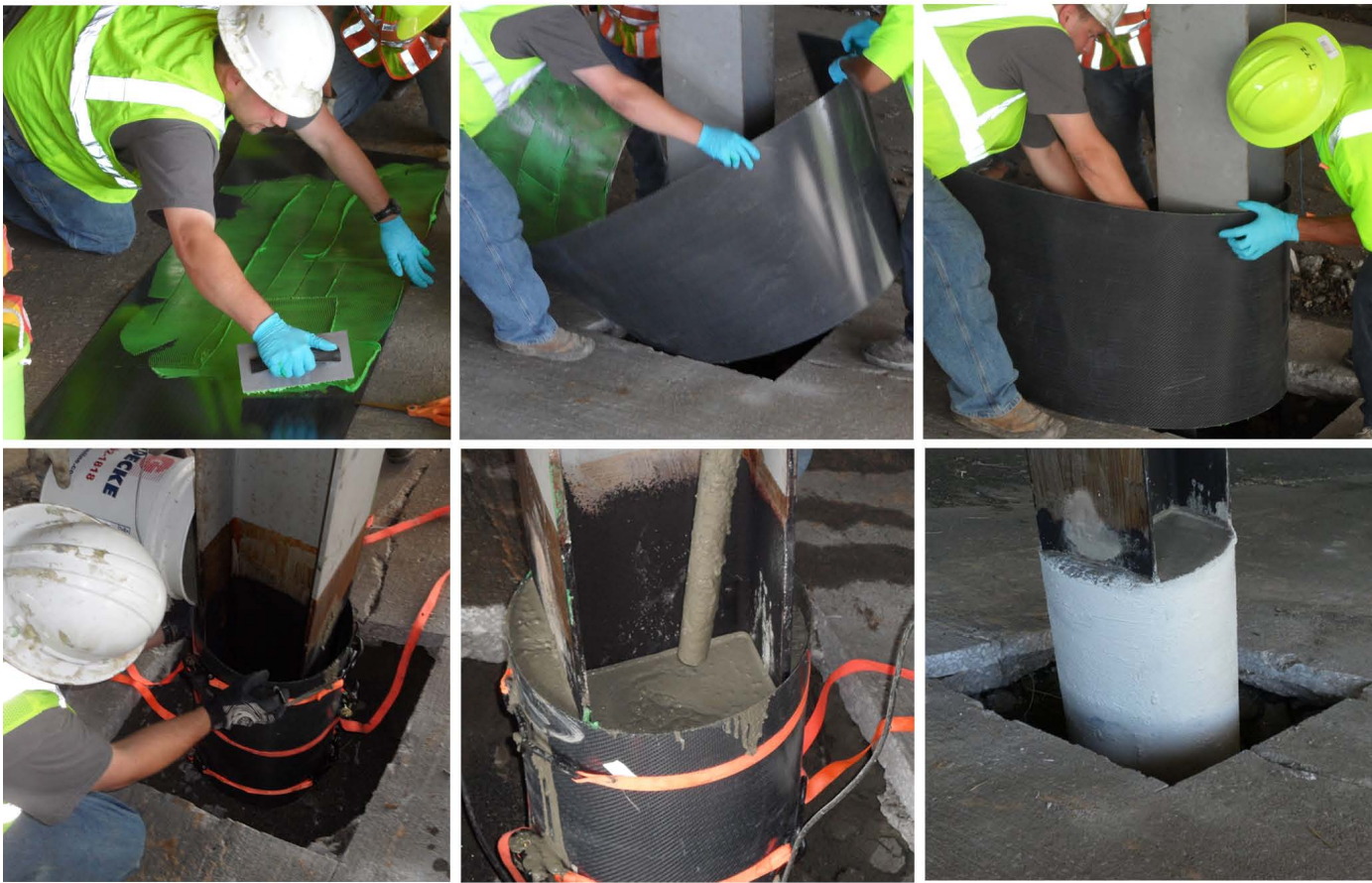
PileMedic installation steps, from upper left: application of epoxy to laminate, creating the shell around the pile, positioning the shell, filling with grout and vibrating, finished painted shell.
