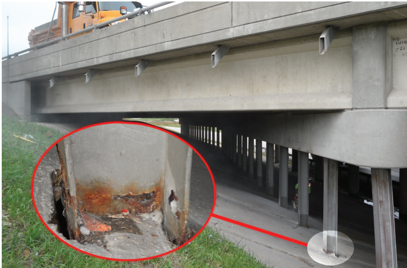
One of the 49 corrosion damaged piles in I-70/I-270 Interchange that were repaired with this technique.
