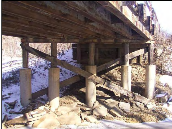
Figure 4.8. Encasing the center piers with concrete for pile restoration (Bridge No. 149 Boone County – February 11 2005)
