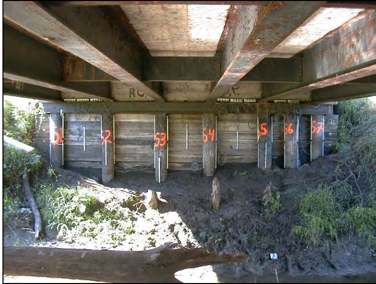
Figure 8.15. South abutment instrumented with strain transducers (Bridge No. 243470 Marshall County – July 27 2005)
