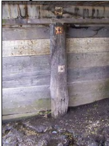
(b) Bulging of timber fibers (Bridge No. 35-87-00 Buchanan County – February 15 2005)
