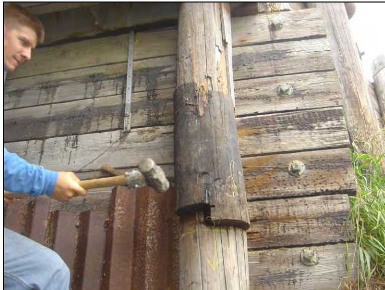
Figure 12.21. Installing a new timber section to repair pile no. 7 (Bridge No. 029070 Humboldt County – July 12 2006)
