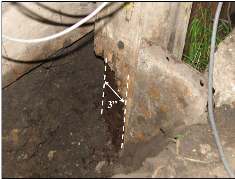
Figure 12.9. Advanced section loss at pile No. 6 at the east abutment (Bridge No. 029070 Humboldt County – July 12 2006)
