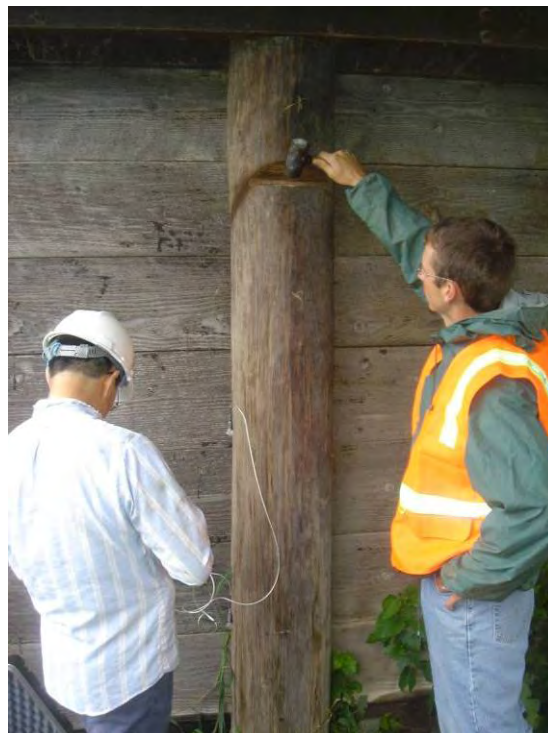
Figure 9.24. Applying an axial impact to the notched pile (Bridge No. 237350 Mahaska County – August 17 2006)
