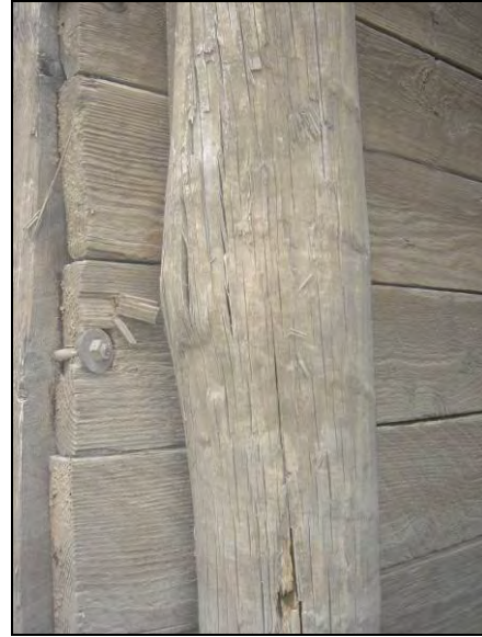
(b) Bulging of timber fibers
