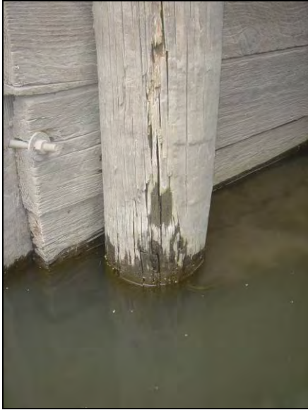
(a) Biological deterioration near the water level
