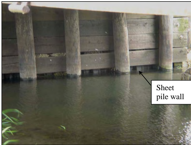
Figure 7.8. Sheet pile wall driven behind the south abutment to prevent backfill erosion (Bridge No. 7710 Boone County – June 1 2005)
