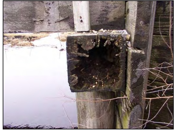
(b) Biologically degraded timber cap (Bridge No. 15-00-62 Buchanan County – February 15 2005)
