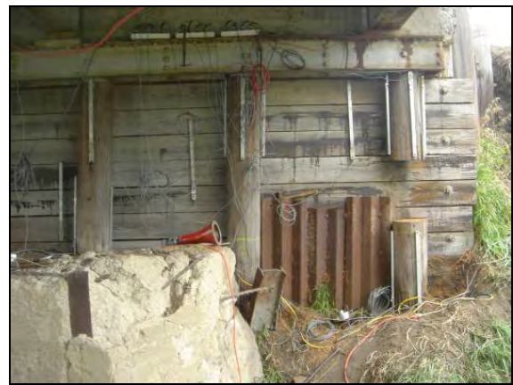
(b) A section of pile no. 7 removed
