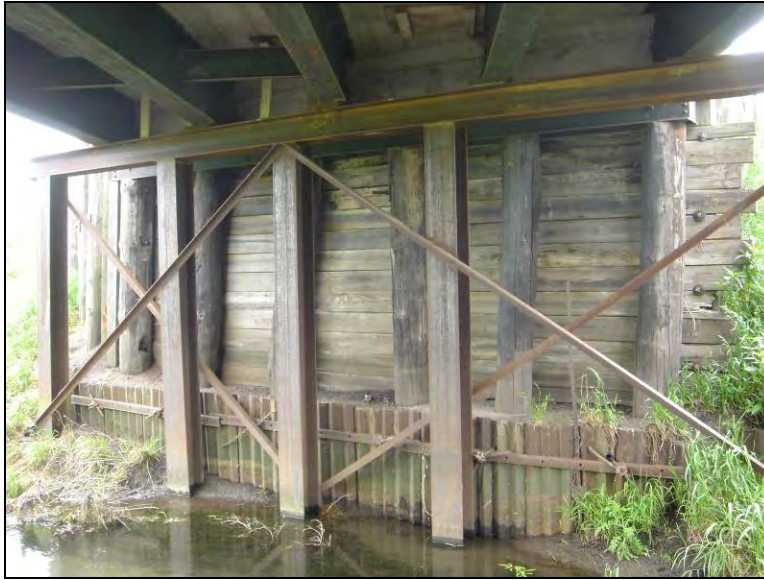
Figure 4.14. Steel piles used to replace deteriorated timber abutment (Bridge in Boone County – June 1 2005)
