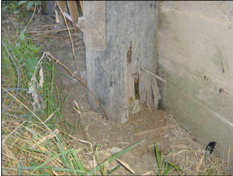
Figure 9.8. Brooming of pile No. 2 near the ground level (Bridge No. 237350 Mahaska County – October 25 2005)
