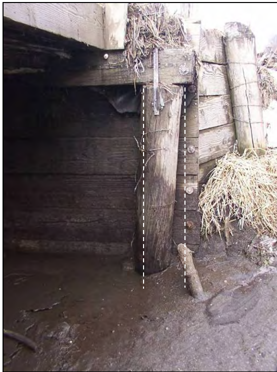
Figure 4.6. Misalignment of a timber pile (Bridge No. 22-00-44 Buchanan County – February 15 2005)
