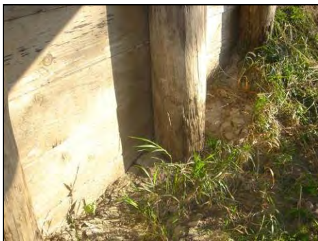
(c) Soft pile section with high moisture near the ground level
