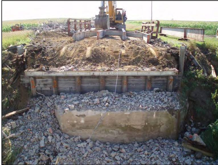
Figure 12.12. Removing the bridge super structure – looking west (Bridge No. 029070 Humboldt County – July 28 2006)
