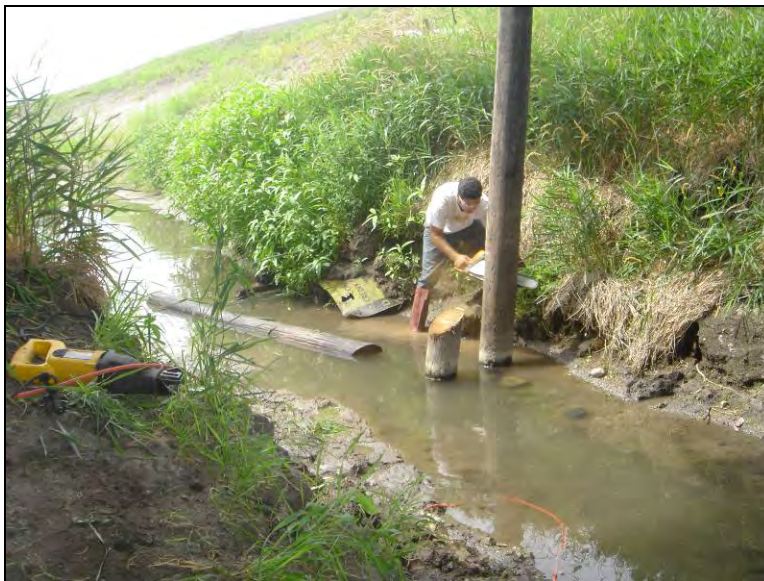
Figure 12.4. Cutting the timber piles supporting the bridge pier (Bridge No. 029070 Humboldt County – July 10 2006)
