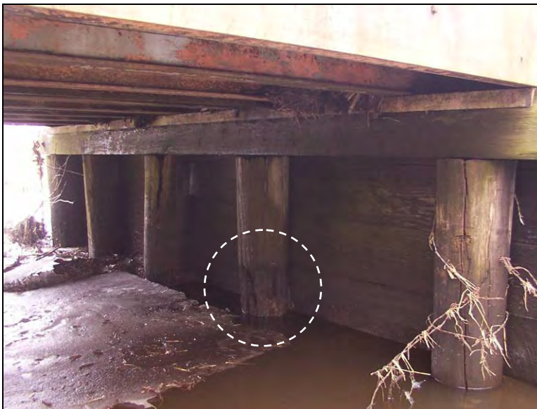
Figure 4.3. Reduction of pile cross section by abrasion from flowing debris and ice (Bridge No. 27-74-23 – February 15 2007)
