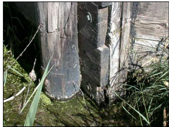
(b) Soft section near the water level
