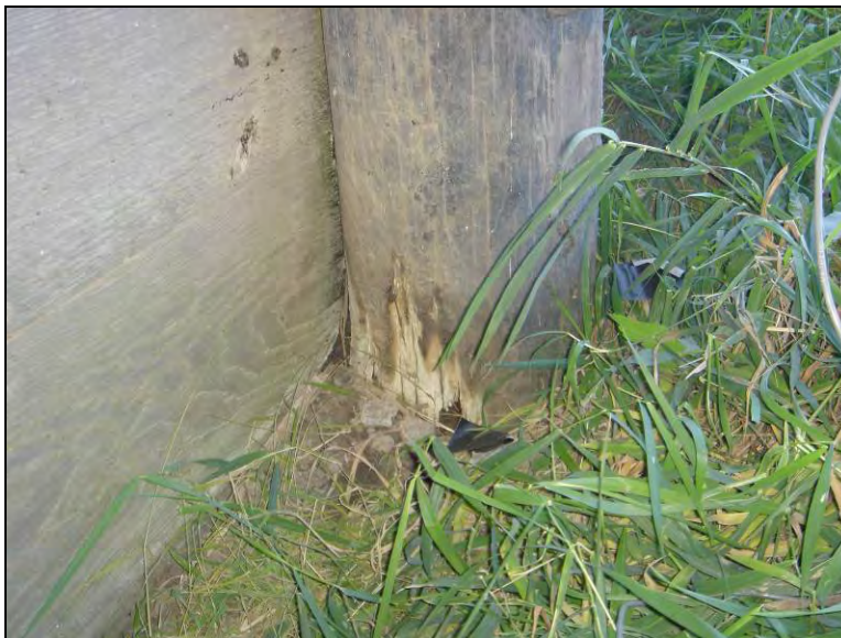
Figure 9.9. Rotting observed at pile No. 5 (Bridge No. 237350 Mahaska County – October 25 2005)
