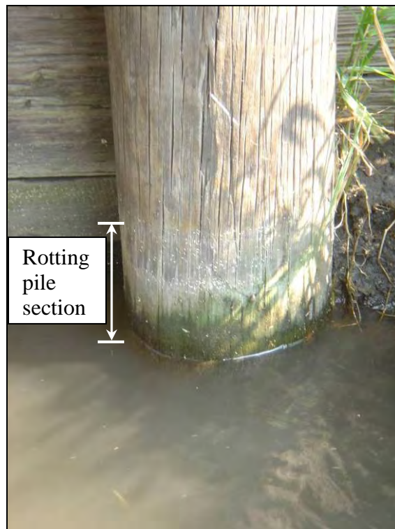
Figure 7.7. Soft section at pile No. 7 above the water level (Bridge No. 7710 Boone County – July 1 2005)
