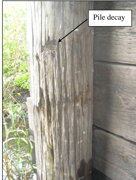
Figure 7.6. Deterioration at pile No. 1 (Bridge No. 7710 Boone County – July 1 2005)
