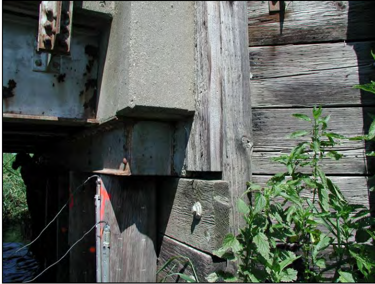
Figure 7.13. Possible eccentric loading caused by misalignment of pile cap (Bridge No. 7710 – Boone County)
