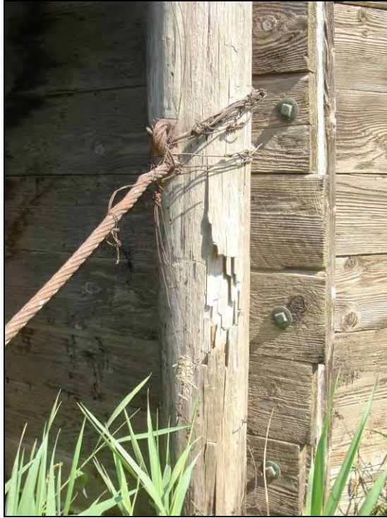
Figure 4.5. Ultraviolet degradation of a timber pile (Bridge No. 23-73-50 Mahaska County – July 8 2005)
