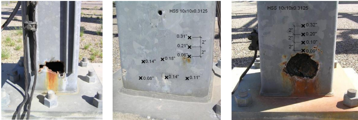
Fig. 1. Typical steel columns damaged by corrosion and measured wall thickness
