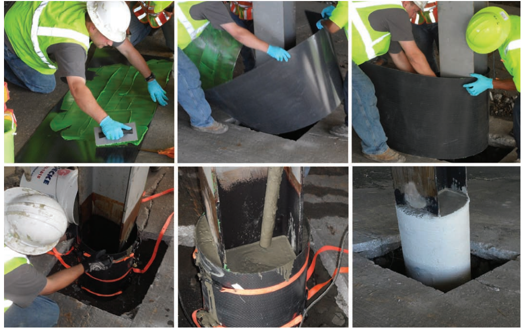
Steps in installation of PileMedic™ clockwise from upper left: application of epoxy to laminate, creating the shell around the pile, positioning the shell, filling with grout and vibrating, finished painted shell.
