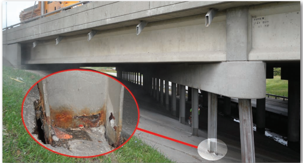
One of the 49 corrosion-damaged piles in the I-70/I-270 interchange (St. Louis, Missouri) that was repaired with this technique.
