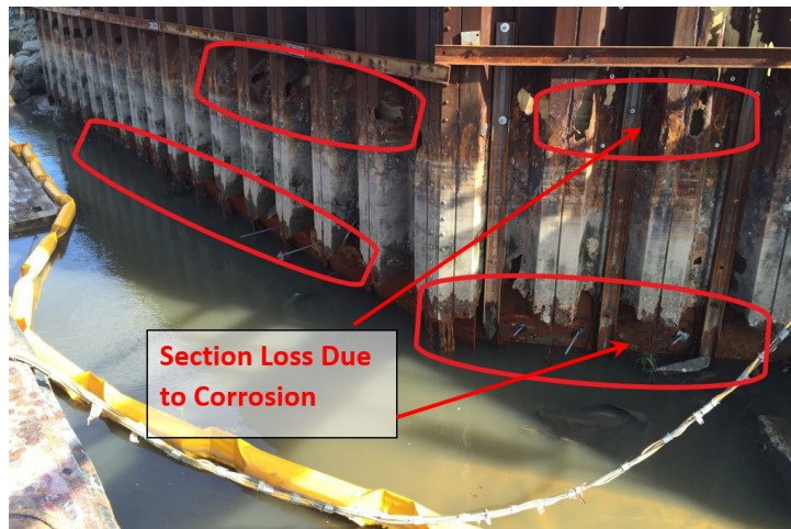
Fig. 1. Corroded seawall with section loss
