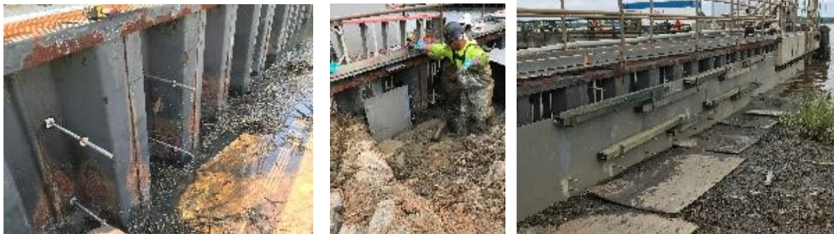
Fig. 3. Steps in repair of a corroded seawall including attachment of J-bolts, placement of GFRP rebar, and connecting the SPIRe® panels and walers prior to placement of grout
