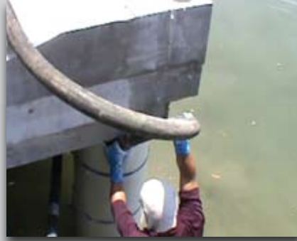
Mix grout and fill the annular space between the jacket and the pile with grout
