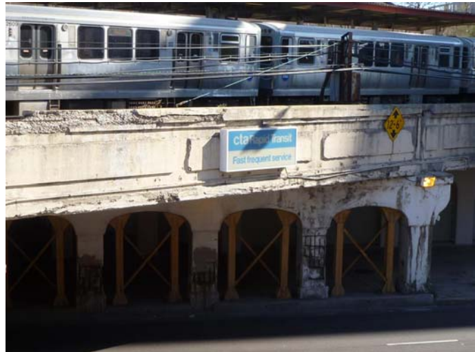
Fig. 1. Corrosion-damaged concrete piles in Chicago being assisted with steel trusses
