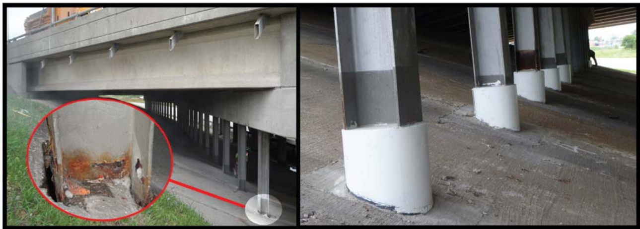
Fig. 4. The I-70/I-270 interchange in St. Louis, MO where 49 corroded bridge piling were recently repaired with PileMedic™ jackets.
