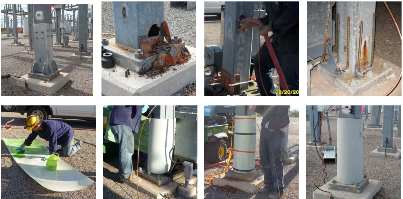
Fig. 3. Repair of steel poles at TEP substations: original repair concept; corroded pole; filling the pole with grout; reinforcing steel welded to base plate; applying epoxy to the laminate, wrapping it around the pole and holding it with straps while grout is placed; finished and painted jacket
