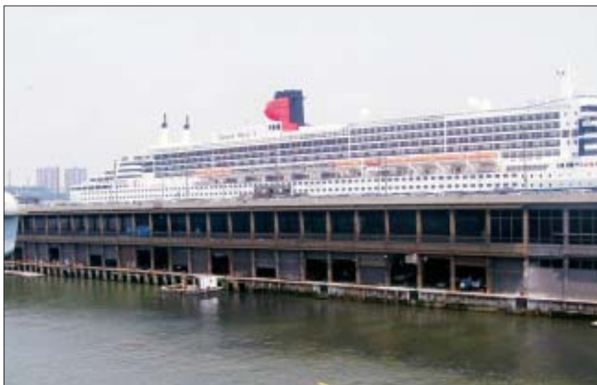
New York City's Passenger Ship Terminal timber piles are being attacked by wood-boring marine worms.
