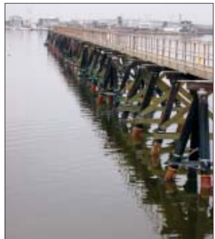
Refurbished wooden piles are now returned to their original strength or better.
