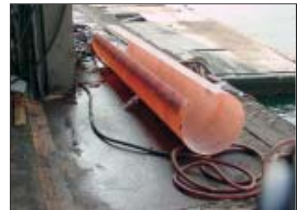
To solve the marine worm problem, an FRP pile encapsulation system was selected.
