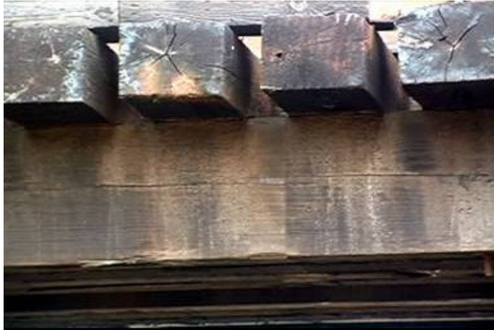
Fig. 2.3 Photograph of horizontal shear crack present in stringer
