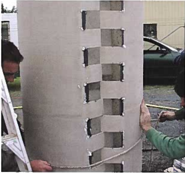
Fig. 2: The 2003 prototype FRP jacket used finger joints bent inward to be embedded in the grout, subsequently placed in the annulus formed between the pile and the jacket
