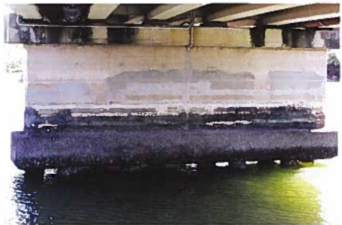
Fig. 1: View of a typical blade pier rising from a pile cap supported on 10 closely spaced PC piles
