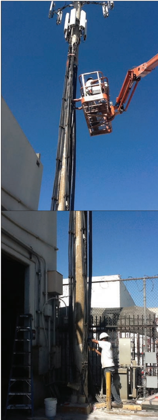
Fig. 1: Overview of the pole and the congested work space available at the base
