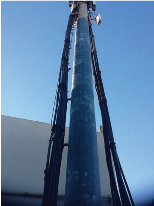
Fig. 4: Carbon and glass FRP applied to the lower 26 ft (7.9 m) of the pole
